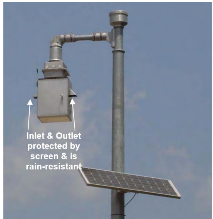
Figure 2. Close-up view of AreaRAE cabinet and solar panel.
